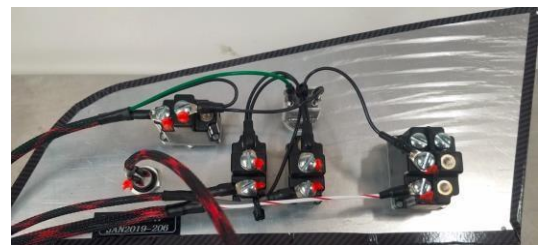
Switch Panel, Back Side
