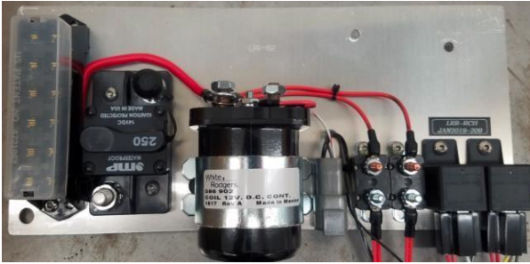
Rear Power Distribution Panel View
